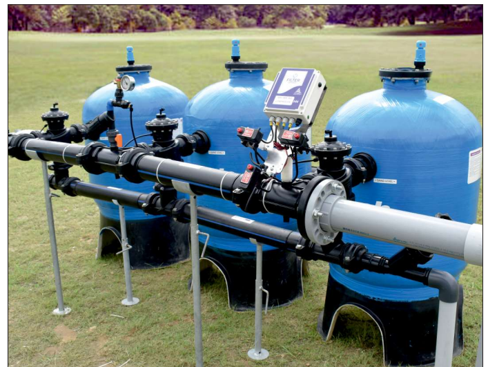
Backflush valve installed with Sand Media Filters
