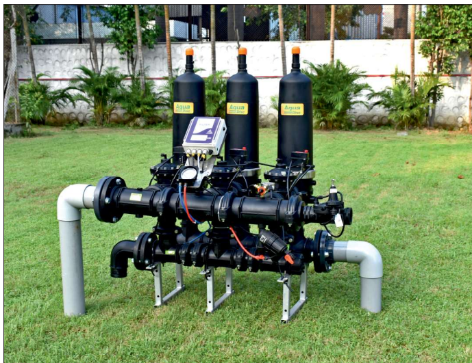
Backflush valve installed with Automatic Disc Filters
